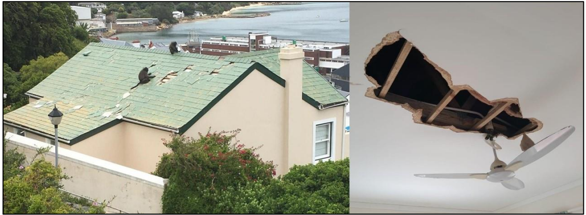
Figure 2. Waterfall troop baboons causing damage to roofs and subsequently ceilings.
